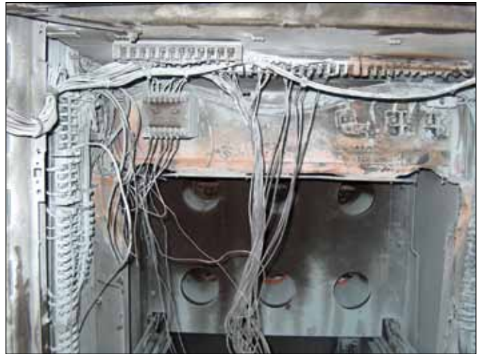
Figure 2 — Damaged 5 kV Circuit Breaker Enclosure
