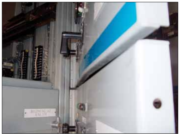
Figure 3 — Damage to Upper Enclosure
