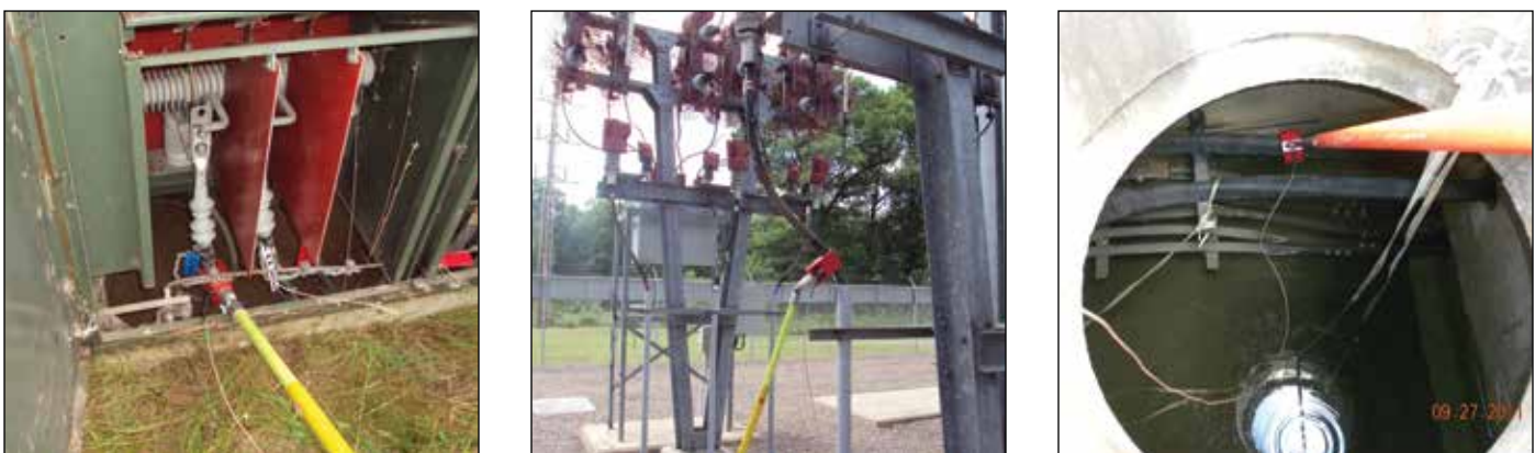
Figure 4: Non-galvanic capacitive sensor is placed on the shielded part of medium-voltage cables for PD measurement.
