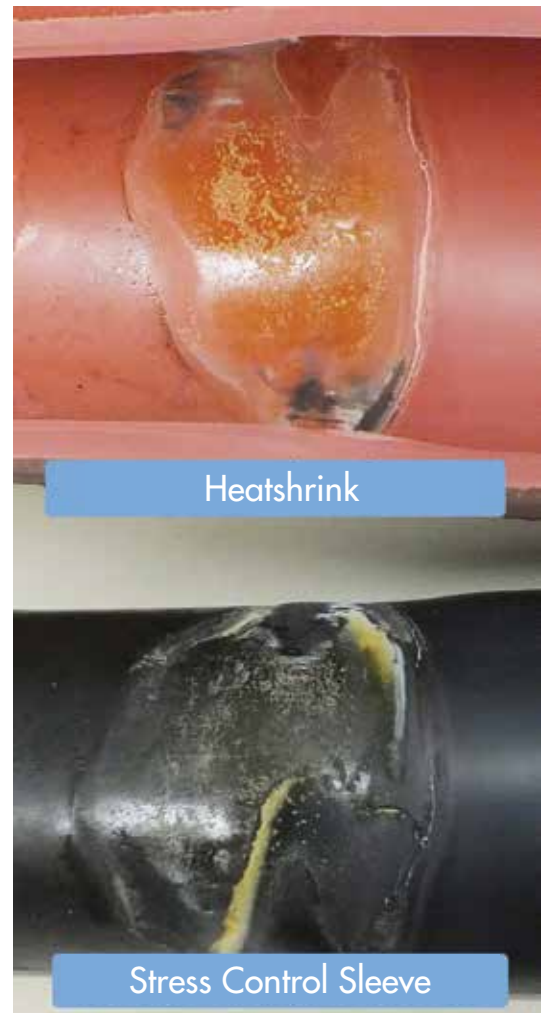
Figure 5: Partial Discharge Location
