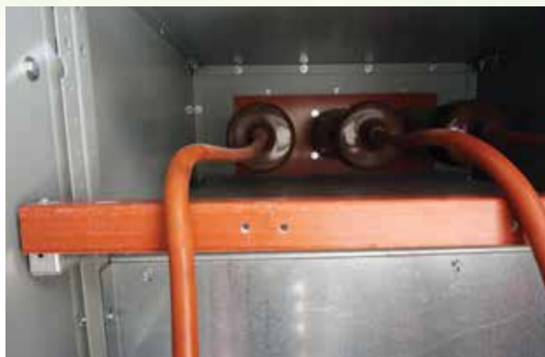
Figure 6: Improperly Installed PT Cables
