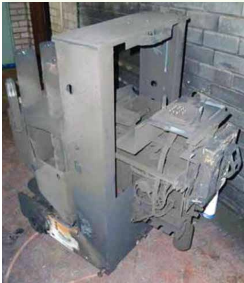
Figure 1: Result of Inaction — Catastrophic Failure
