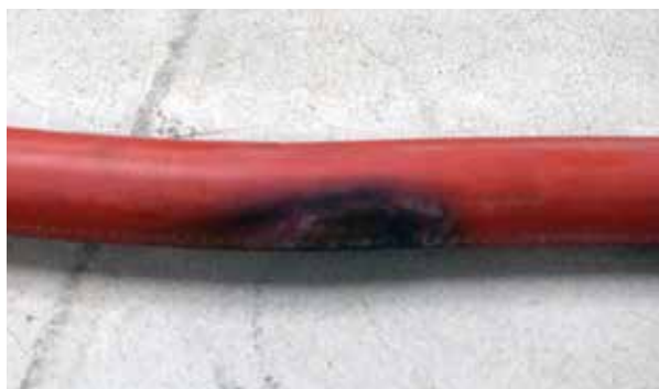
Figure 8: PD Damage to PT Cable
