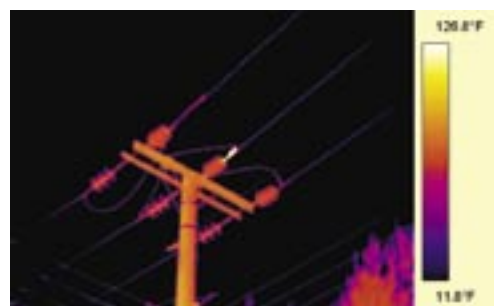
Figure 8 — Properly thermally tuned for finding problems.
