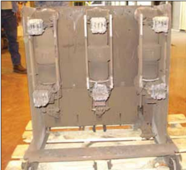
Figure 6 — Severe Breaker Damage Caused by Improper Rack-In Operation
