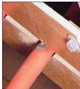
Figure 2 — Unshielded Medium-Voltage Jumper Cable
