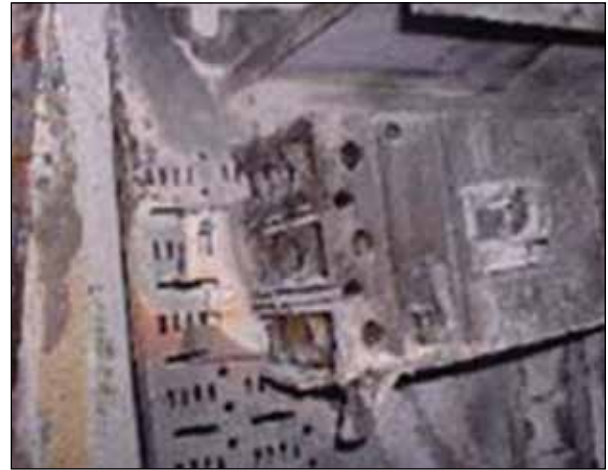
Figure 7 — Severe Damage from Arcing Ground Fault
