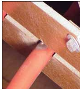
Figure 2 — Unshielded Medium-Voltage Jumper Cable
